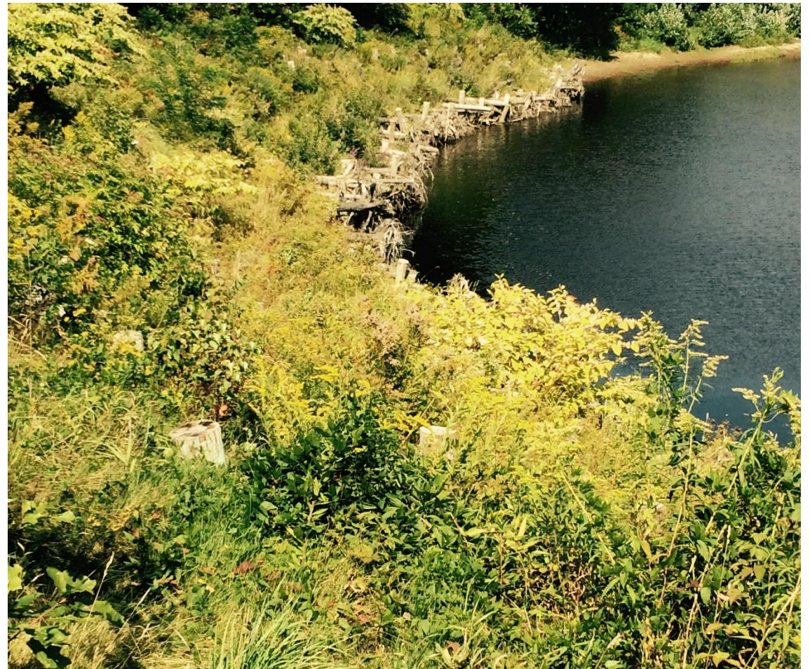
Sandy River Bank Stabilization, Farmington Falls, Maine. Land and Water Magazine September/October 2016. Peter Hanrahan, CPESC
